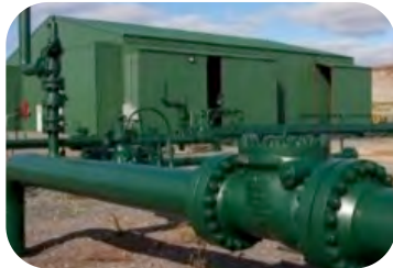
Compressor and Pump Station Noise
