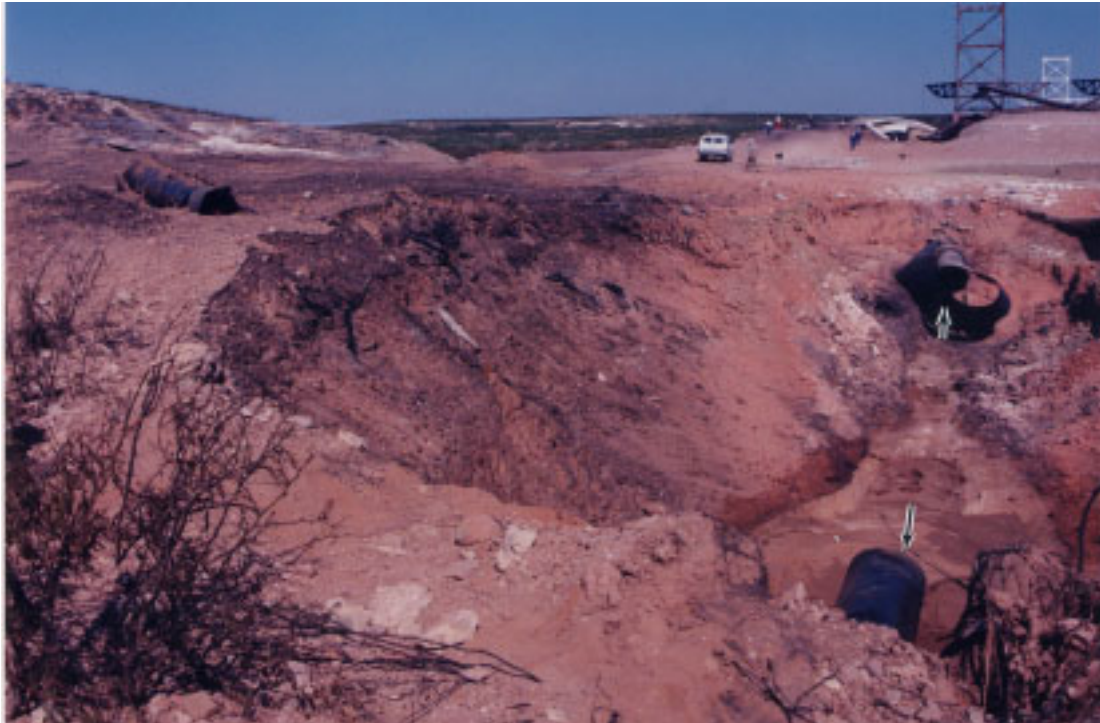
Figure 6. Looking west at a portion of the crater created by the rupture. The missing section of pipe between the arrows was ejected from the crater.
