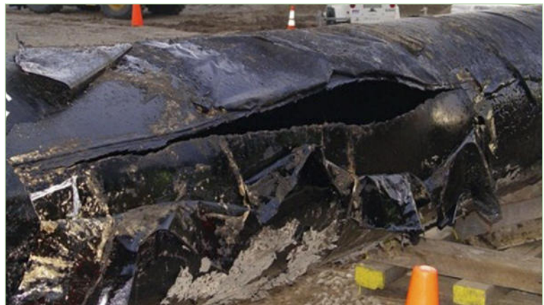
The Enbridge pipeline that failed in Michigan in 2010 had older enamel wrap coating installed
