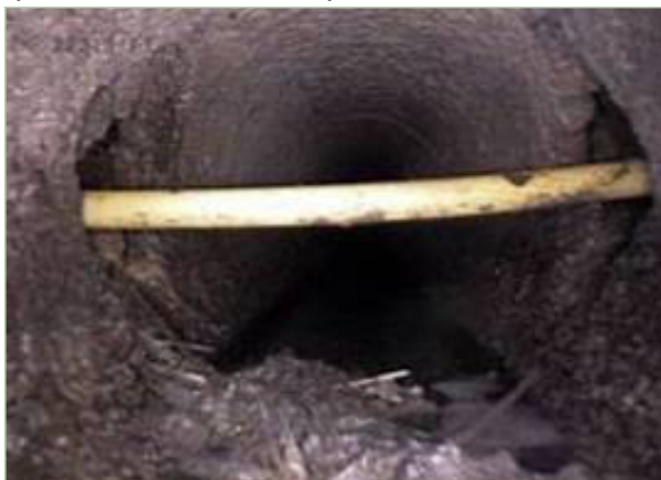
Example of a problematic cross bore of a gas pipeline through a sewer line
