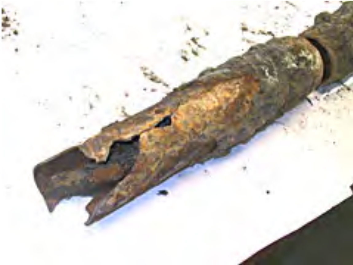
Damaged cast iron piping
